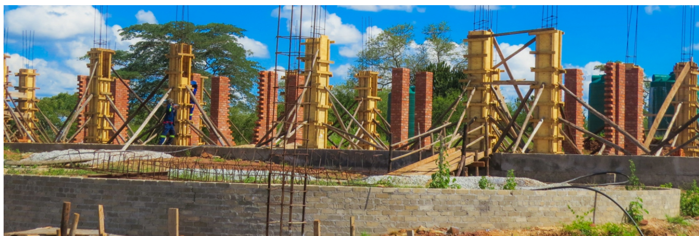
Construction of the Administration Block and Laboratories at the Innovation Centre for Dryland Agriculture (ICEDA) in Chivi was at 23% at the end of 2022
